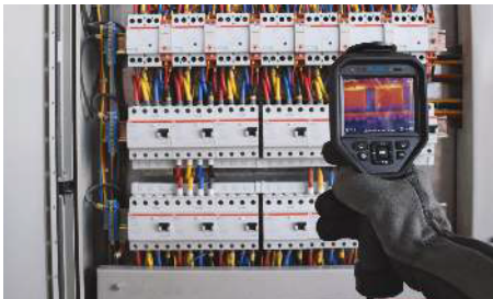
Electric Panel Inspection
